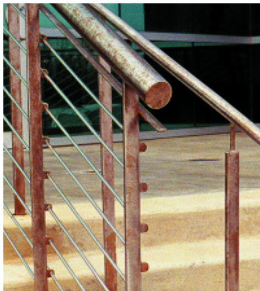
Figure B Type 304 stainless steel with a rough finish was the wrong choice for handrails exposed to deicing salt laden road mist. Cleaning will remove the staining but it will reappear every year. (Photo credit – TMR Stainless)
